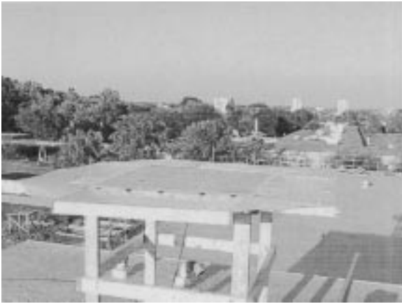
Fig. 10. Array as built. View is slightly North of East.
